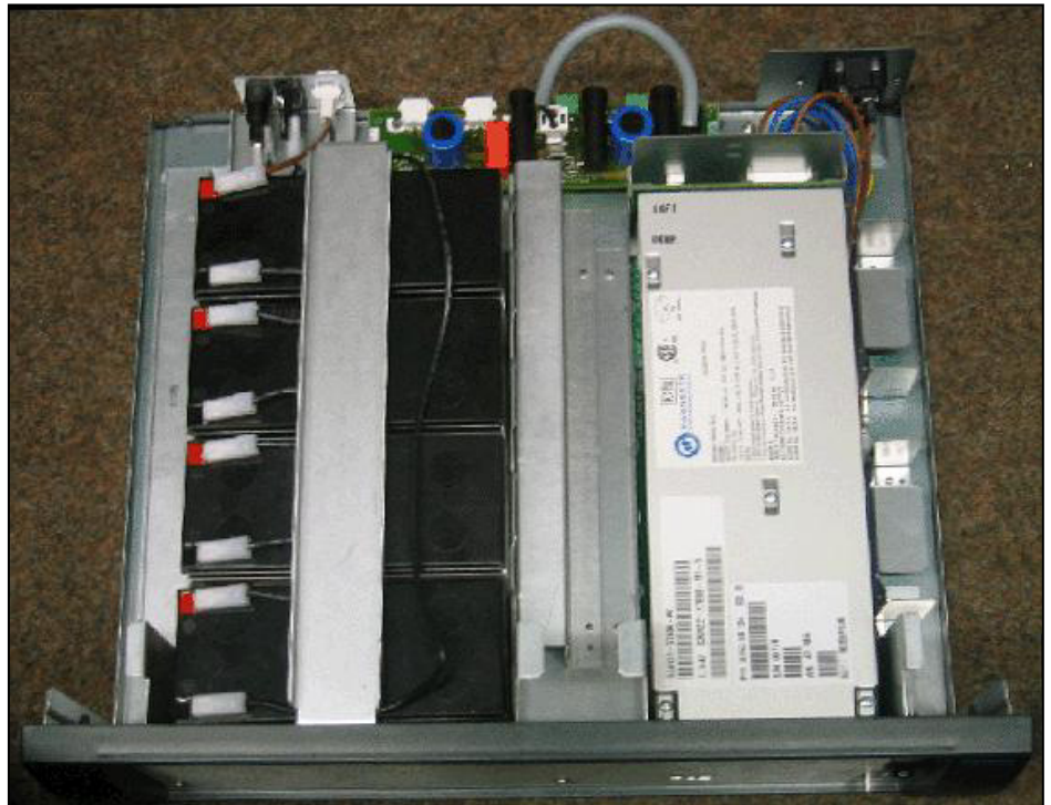
Figure: OpenScape Business Powerbox – Equipped with four 12V 7Ah batteries and LUNA2 power supply
